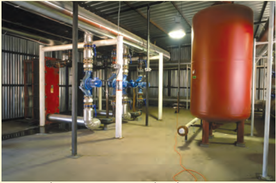
Heat exchangers, pumps, and tank at Masson Radium Springs Farm geothermal greenhouses. Heat exchangers are used to transfer heat from geothermal water to a closed-loop fresh water heating system.
